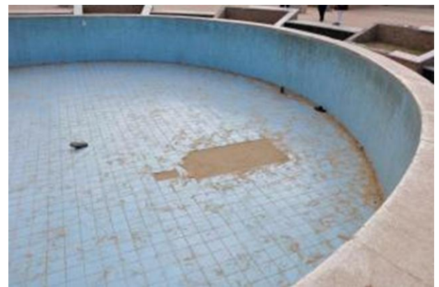
Central Fountain at Brotherhood Park before maintenance
