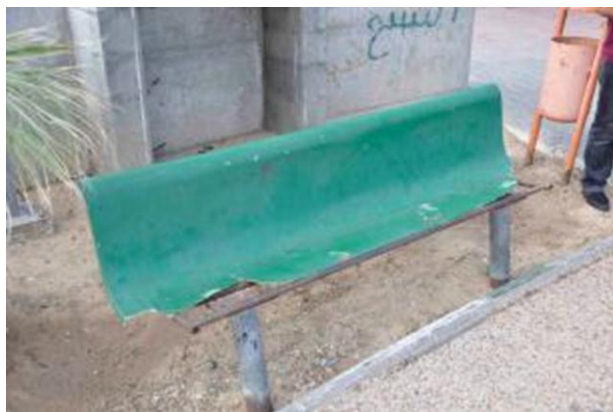
Benches at Brotherhood Park before maintenance
